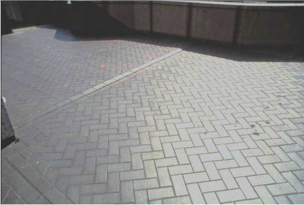
dark brick pavers, set in mortar, undersized expansion joint
