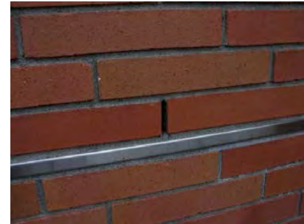
Weep detail. College of Engineering, Portland State University, Portland, OR, ZGF Architects
