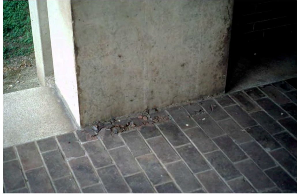
dark brick pavers, set in mortar, no expansion joint
