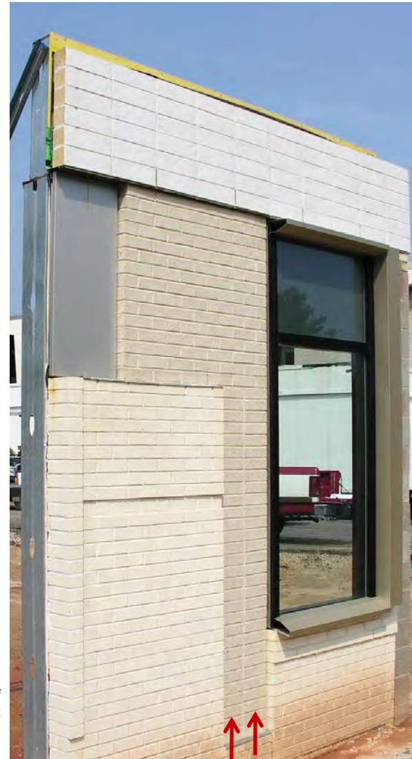
Anchors or ties are installed at edges of veneer panels, and at greater frequency in stackbonded panels
